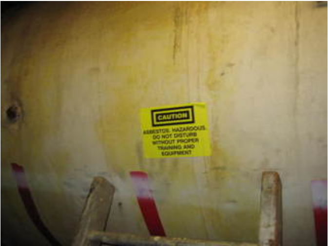
Hazardous Material- $1.9 M
