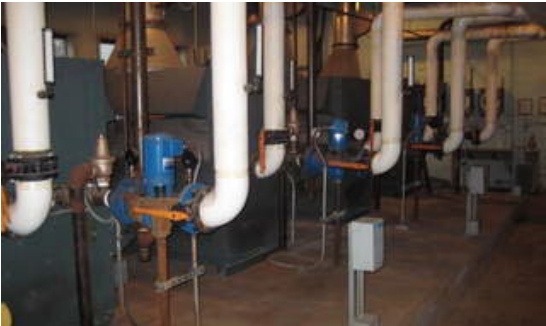
Two-pipe non compliant HVAC system - $10.3 M
