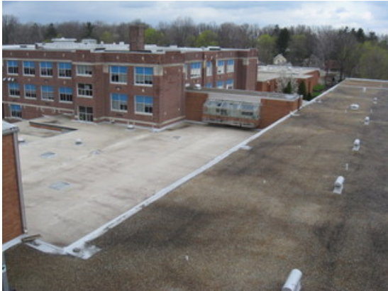
Leaking /aged roofs- $3.3 M
